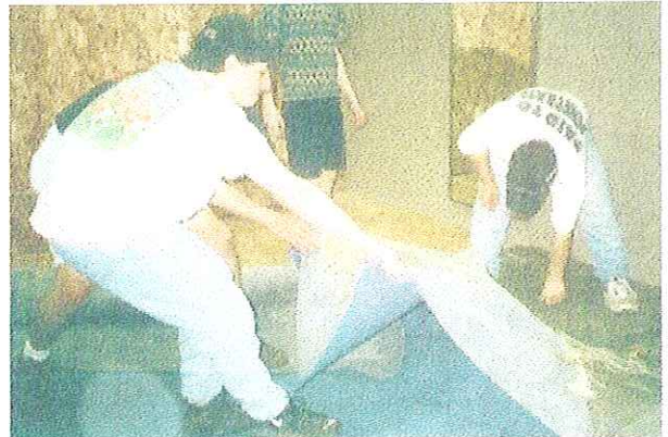
Volunteers from Clarion U. apply glue and place carpeting in the weight room.
