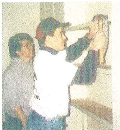
A volunteer from Clarion University turns an unneeded doorway into built-in bookshelves.
